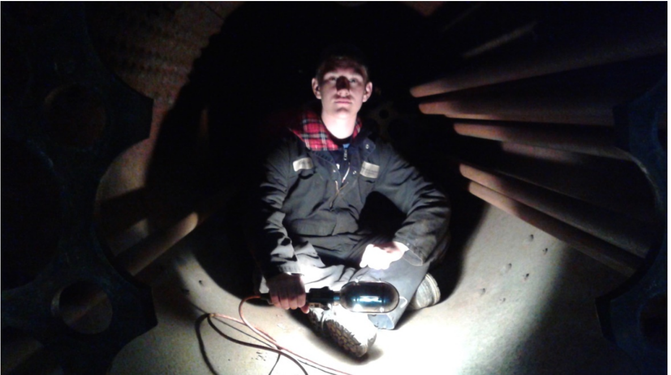
Peter Leis inside Main Barrel after removing most of the tubes and flues. (Photo by Stephen Leis)
