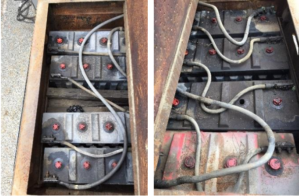
Different battery sizes between engineer and helper's side.
