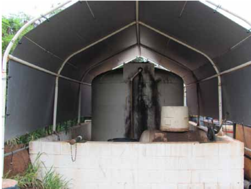
2000 Gallon catchment Tank for Oily Water
