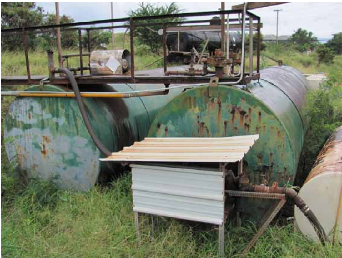
2- 10,000 Gallon Tanks for diesel fuel and waste oil
