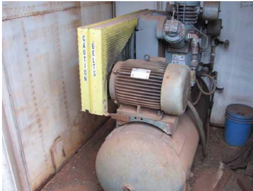
Shop Air Compressor
