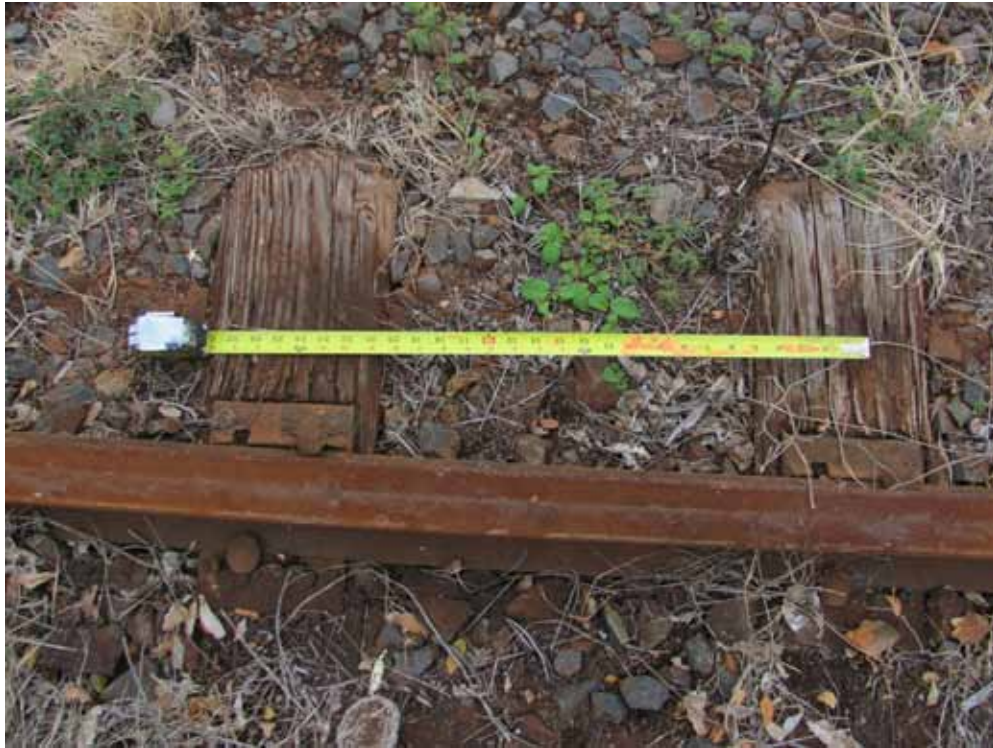
Track Section with ties measured out on 24" centers for steel OTM calculations
